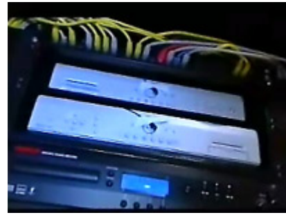
Three boxes in the control room are the hub of the system
